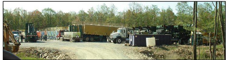
View of the Little 1H / Little 2H well site location in Snow Shoe Township, Centre County, showing the on-site activity just prior to completing the hydraulic fracturing process (commonly referred to "fracing"). Two Marcellus Shale wells are located here. The depth of the wells is approximately 8000 feet.
